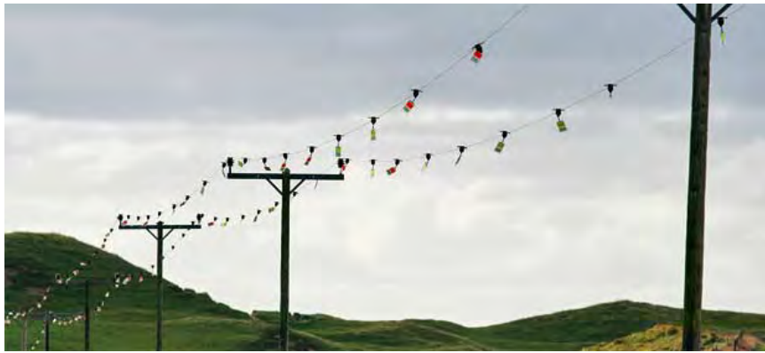
Figure 6.1: Example of bird flight diverters installed on an electric power line.
