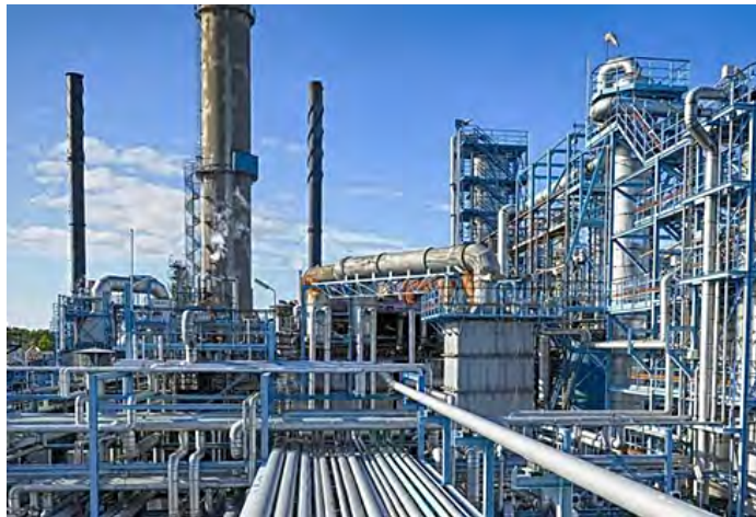
Figure 5.1: Cluttered industrial environment with many pipe arrays.
