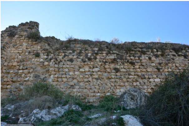
Figure 22: Photograph of the current state in detail of the pathologies suffered by the castle.
