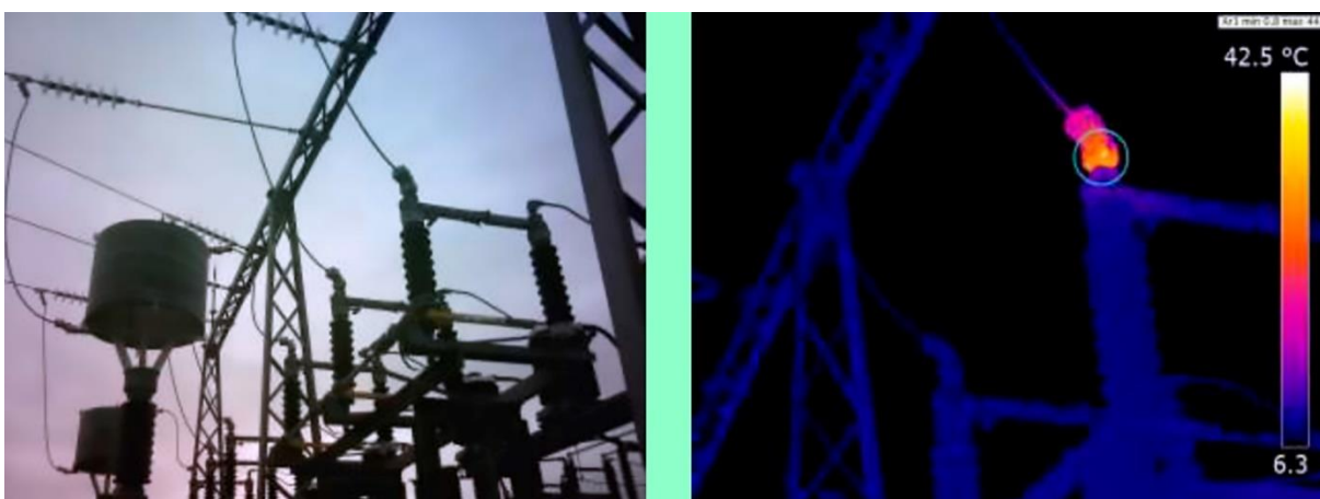
Fig. 5. Visible and infrared images of a hot spot in a 66 kV disconnector.
