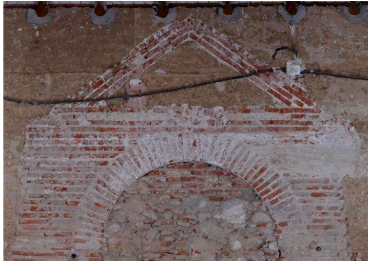
Figure 14. Detail of the front and the semicircular arch of the new open portal on Facing 2.
