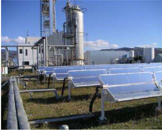
Fig. 1. ACUREX collector field (courtesy of PSA).
