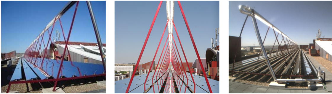
Fig. 4. Linear Fresnel solar collector installed at the Engineering School of Seville (Spain).
