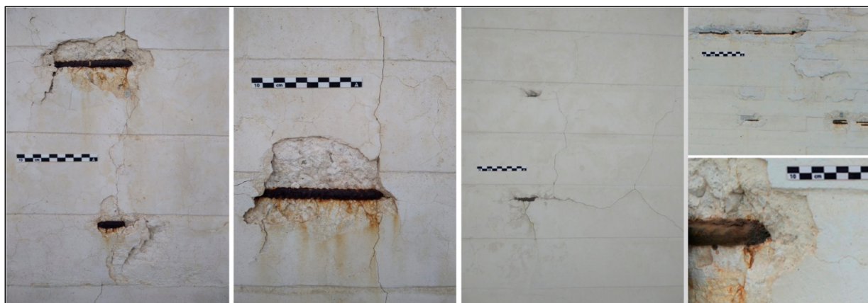
Figure 2 Close-up of alterations in the exposed reinforced concrete façade: detachments, shrinkage cracks, reinforcement corrosion, oxidation patinas.
