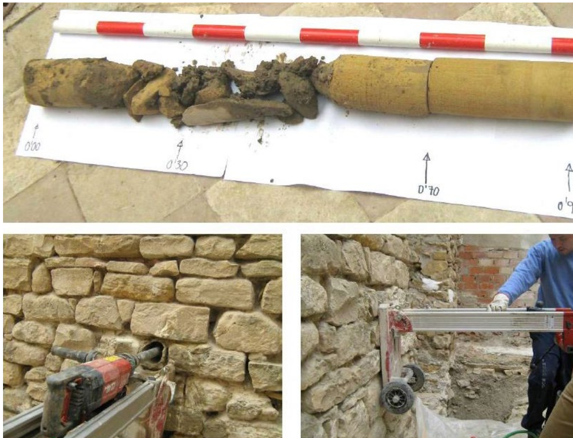
Fig. 6. Test about the internal composition of the façade of the Royal Butchers (16th century) in Porcuna, during the restoration process. It is possible to observe that the façade is characterized by an orderly configuration, instead the “soul” of the wall is composed of filling material without any consistency. (Source: Millán, 2014).
