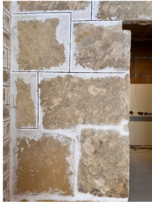
Fig. 5. Detail of a partition wall of losetas (blocks on “sailor” courses). (Source: Belmondo, Millán, 2022).
