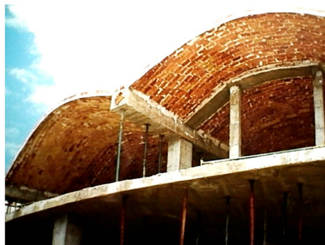
Figure 3. Vault pieces constructed in hollow thin brick by the authors, in Seville.
