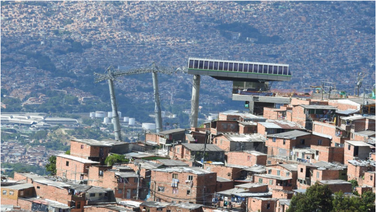
Figure 3: Medellín: A Metro.cable station under construction. Source: By ALONSOZAR [CC BY-SA 4.0], from Wikimedia Commons
