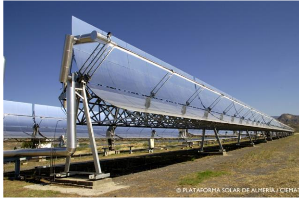
Figura 4. Central termosolar CCP
