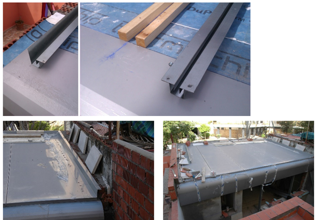
Figure 15. Side edge and centre guides. Assembly process of the coating sheets. Factory-edged finish. Photographs: authors.
