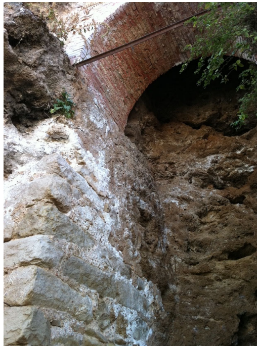
Figure 8. Detail of the pathologies caused by the use of uncontrolled materials. Photo details of the Torre del Reloj [taken by the authors].
