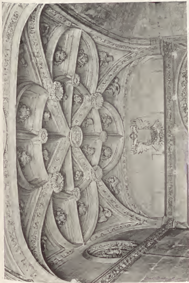
CASAS CAPITULARES. DETALLE DEL TECHO DEL VESTIBULO THE CHAPTER HOUSE. DETAIL OF CEILING OF VESTIBULE
