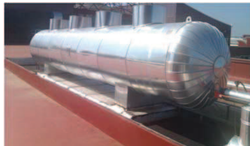
Fig. 3.3. PCM storage tank.
