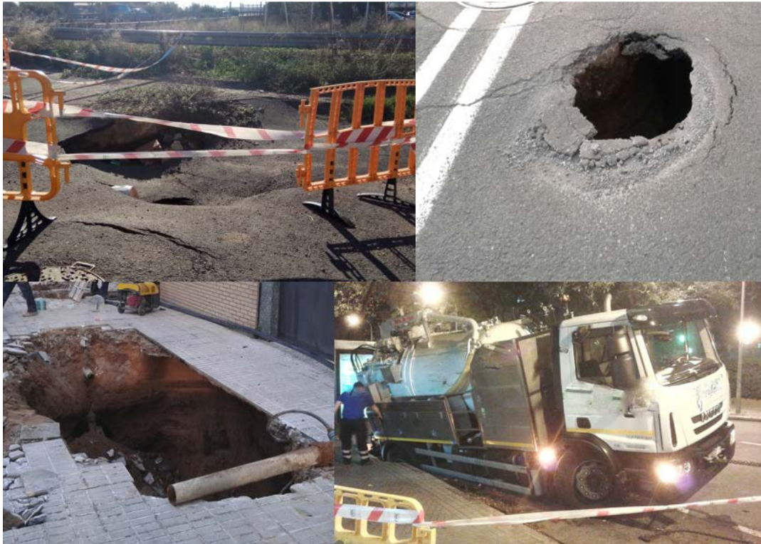
Figure 1. Real consequences of unexpected pipe failures (photographs taken by the authors)
