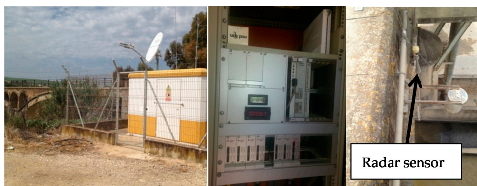
Figure 2. A17 Genil-Écija checkpoint booth with satellite dish for satellite connection with Hispasat 1ª, SAIH equipment (SAINCO/Telvent) and the Vegaplus 62 radar sensor.
