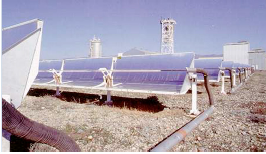
Fig. 1. ACUREX distributed solar collector field
