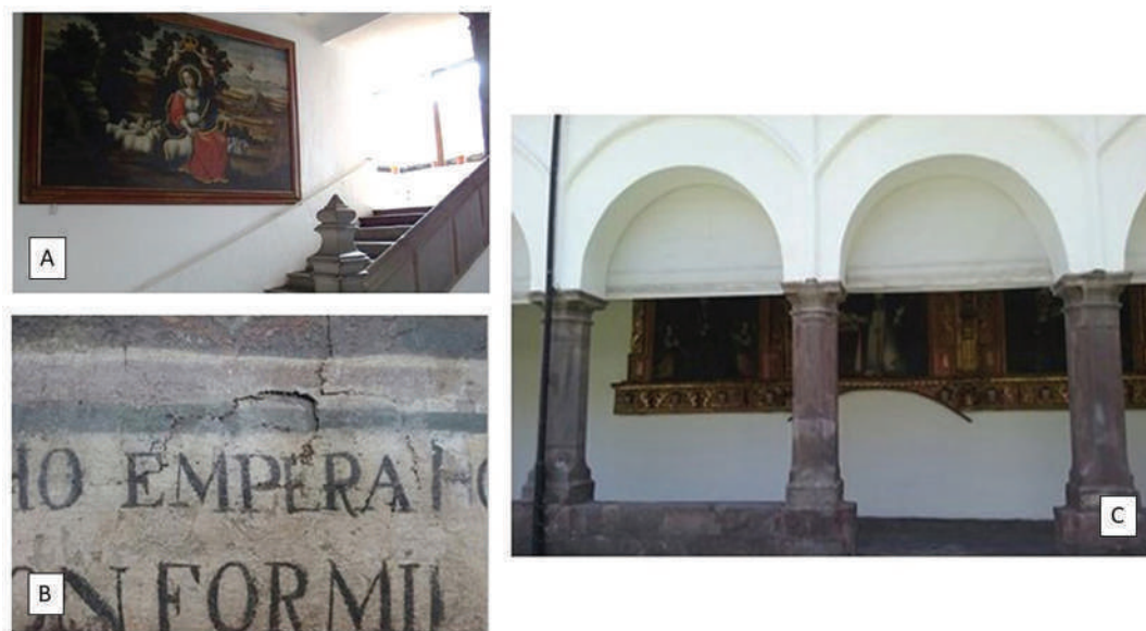
FIG. 6: (A) Location of the painting SC1. (B) Details of the damage caused by sunlight in the pictorial materials and polycromy in SF1. (C) Sunshade system installed in the cloister of Santo Domingo.
