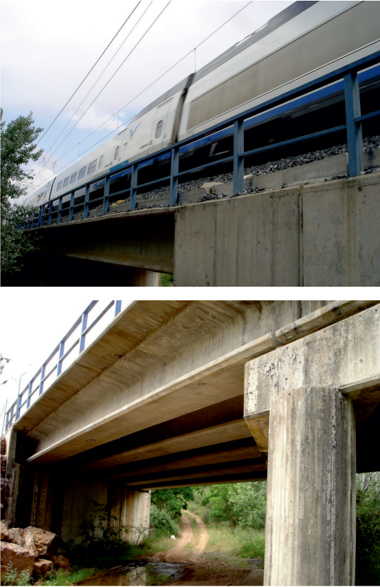
Figure 1: Railway bridge in Spanish high speed line composed by short simply-supported bays
