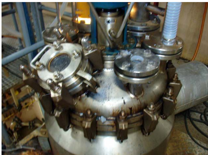
Figura III.63. Reactor de lixiviación (R-3) (vista exterior)
